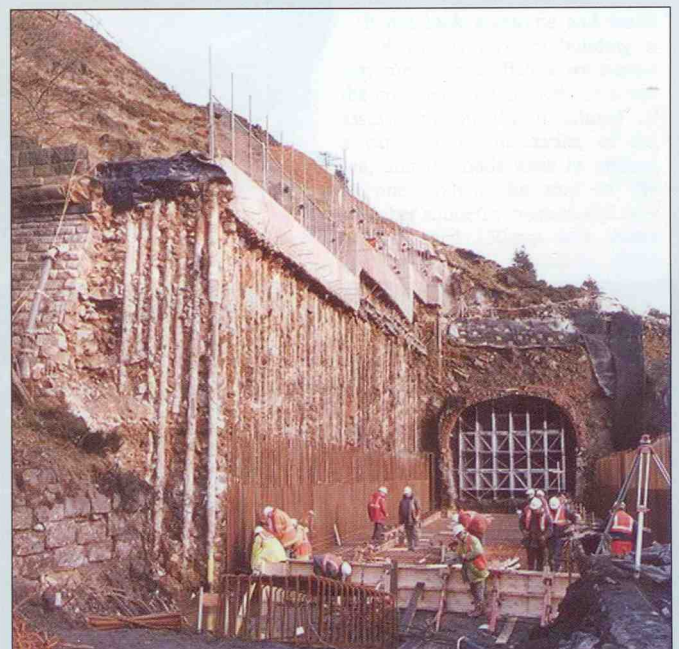
Stabilising the railway embankment at Todmorden for the Horsfall tunnel, 1997-98 (above) and minipiling at the same project
